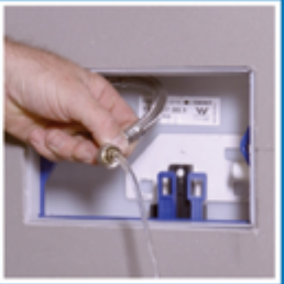
Flush water supply
