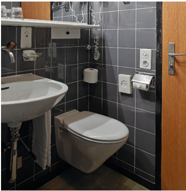
Concealed Cistern installed in 1964 at Hotel Eiger Switzerland
