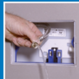
Flush water supply
